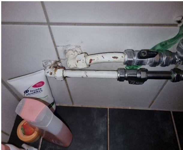
Leaky penetration in shower.
