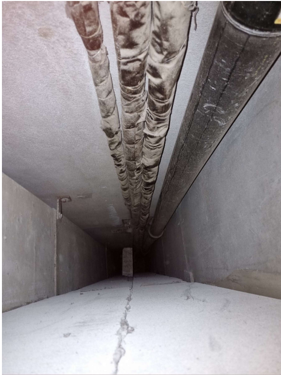
Poor insulation and clamping
