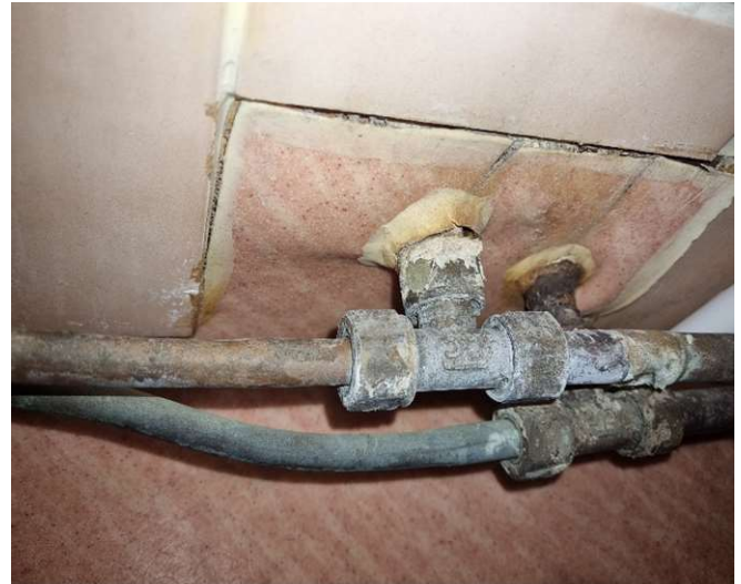
Leaky penetration in shower.
